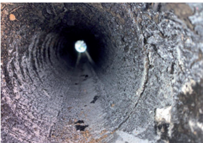
Old asbestos cement pipeline DN 150 with damaged inner layer
