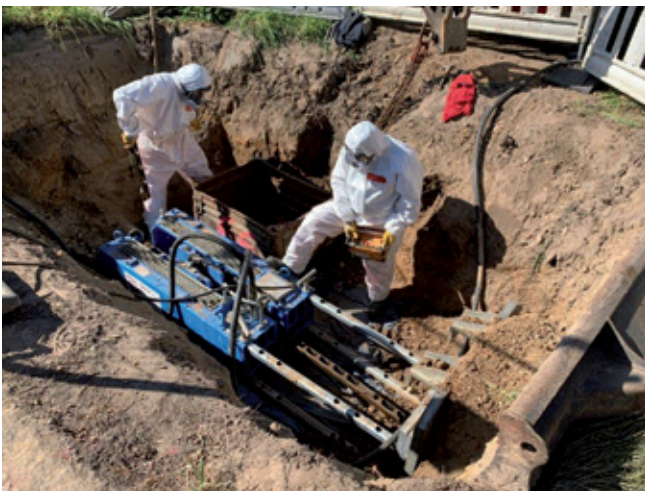
Machine pit with Grundoburst 400 G static bursting rig during the insertion procedure. Compulsory protective clothing for the operators in compliance with TRGS.
