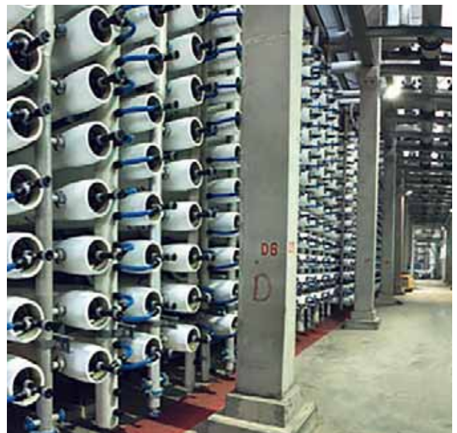
Plastics play a key role in the production of drinking water at seawater desalination plants
